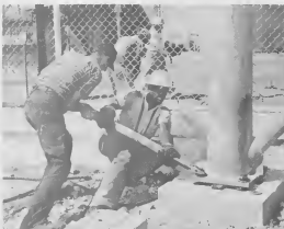
COLUMNS WERE bolted to concrete pads anchored deep in the coral, and were fabricated out of twelve-inch pipe. Workmen apply leverage to a wrench in the operation. COLUMNANAN A wordé firmá cu bolt ariba plachi di concreto hancra hundo den e coral y a wordé fabricá di tubo di dies-dos-dum.
